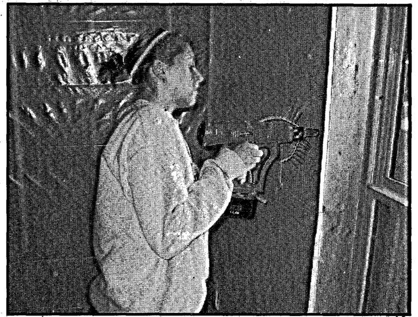
Wayne State College student Allison Friedmann installed drywall at the HFH house on Saturday.
